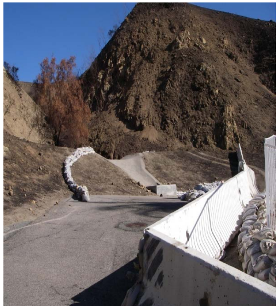
Use of K-rail to channel future debris flow around homes.
