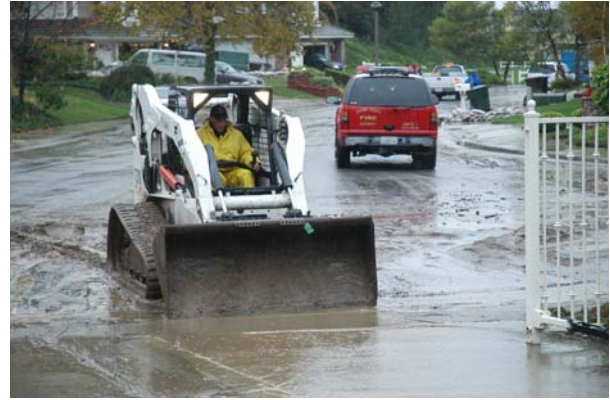
Dozer clearing mud off the street following the rains that hit the fire consumed areas of Yorba Linda.
