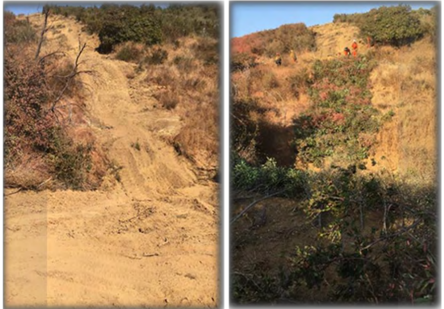
Before and after pictures of the slope erosion control adjacent to a watercourse where crews used cut debris to help regulate and capture sediment
