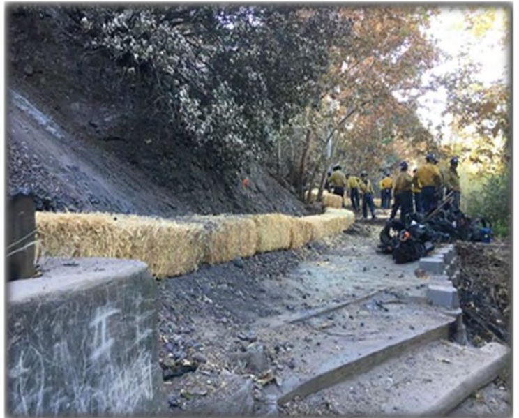
OCFA Hand Crew installed hay bales at the bottom of the slope to control erosion
